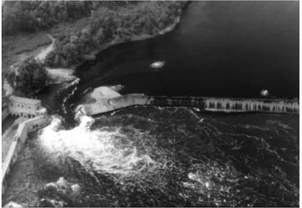
July 1: A section of the coffer dam is removed by an excavator bucket christened with a bottle of champagne. The trickle of the Kennebec quickly increases to a torrent as it erodes the gravel dam and roars through the Edwards breach.
